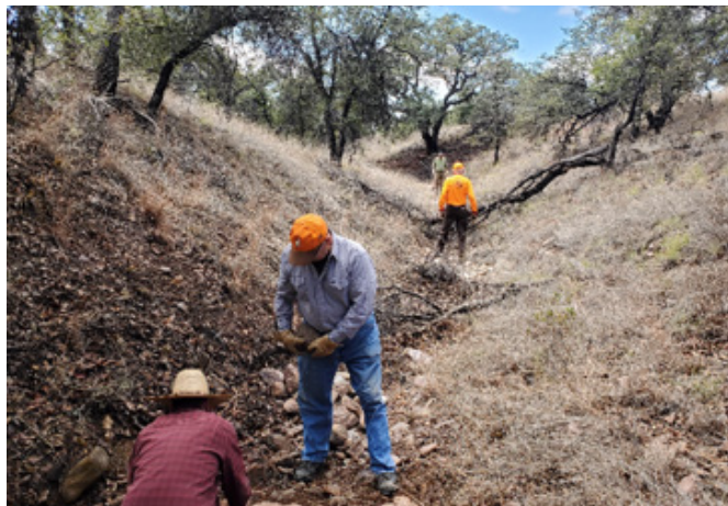
Working with SAQF, volunteers construct loose-rock check dams to slow rainwater runoff and allow water to infiltrate into the soil.
