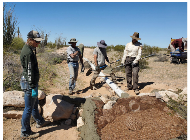
Volunteers help YVRGC construct a wildlife water catchment and storage system near Hat Mountain.
