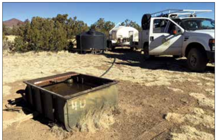
A new storage tank installed on the Pat Springs pipeline to provide additional water storage.
