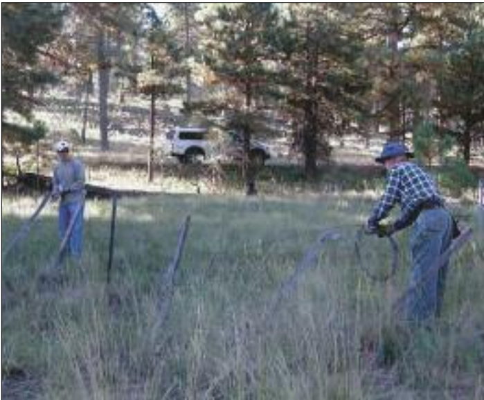
Volunteers removing old fencing near Sinclair Wash and the Arboretum in Flagstaff
